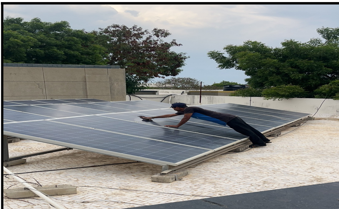
SOLAR PANELS OF 50 KW ON-GRID i.e. NET METERING
